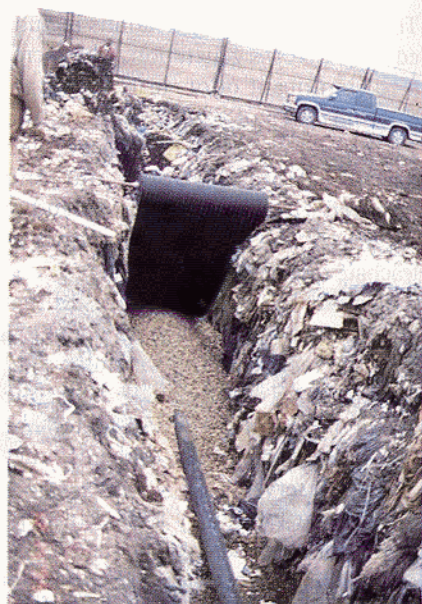
To recirculate leachate, Superior installed horizontal trenches, which then were covered with a light geotextile and backfilled with the excavated waste.
